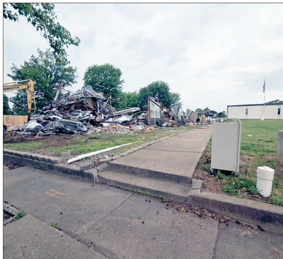
Demolition is underway at the Monett School district's South Building. The building is now set to be replaced with addition parking for the upcoming school year. Jessica Breger/Special to the Monett Monthly
