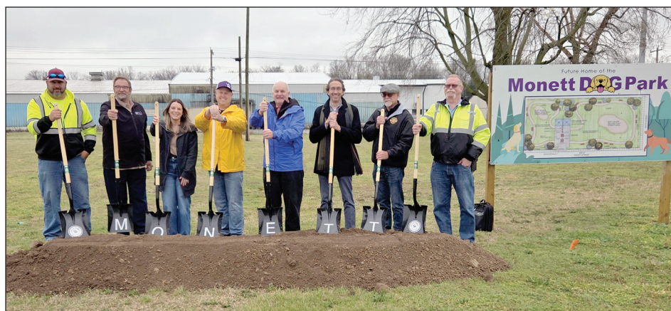
Monett Main Street President Alyssa Vaughn, Commissioner Darren Indovina, Mayor Randy Burke and Commissioner Ken Gaspar were joined by members of The City of Monett and Monett Main Street, along with the Monett Area Chamber of Commerce to break ground on the city's new dog park at 901 E. Broadway St. Jessica Breger/Special to the Monett Monthly
